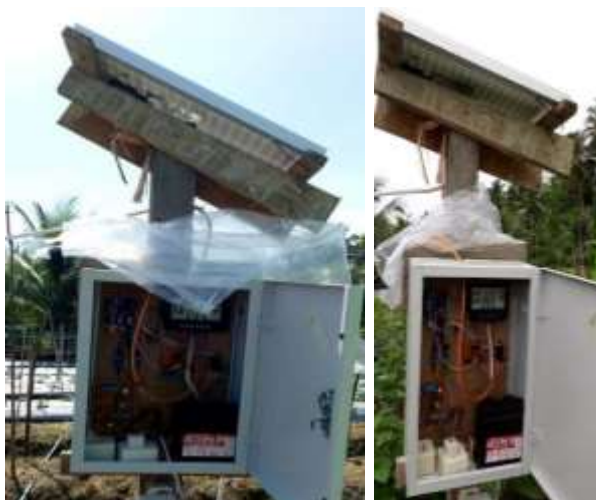
Gambar 5. Panel Sistem Kendali
