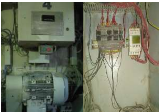
Gambar 6. Kontrol Panel Redlion [6]
