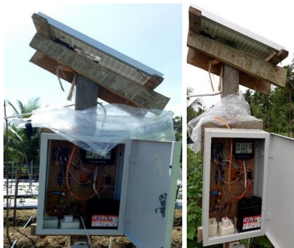
Gambar 5. Panel Sistem Kendali
